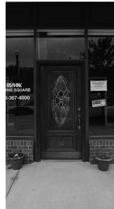
Using a residential door on a commercial building detracts from the overall character of the storefront.
