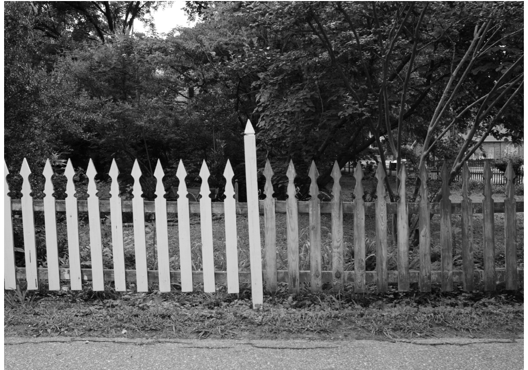
This is an example of an acceptable wood picket fence. However, the fence is also in need of upkeep.
