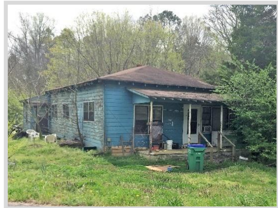
SUBSTANDARD HOUSING OFF SYCAMORE STREET
